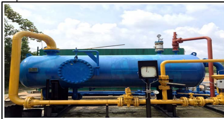
Gambar 2. Separator di Oil Plant SG-09
