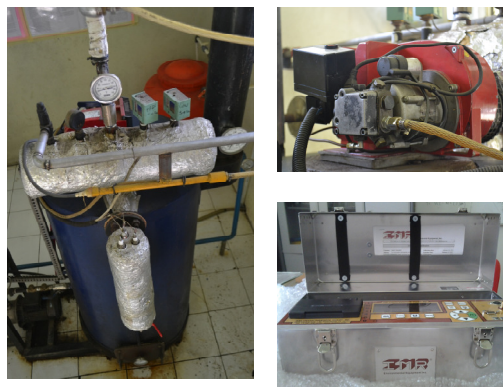
Figure 1. Boiler, Oil Burner and Gas Analyzer
